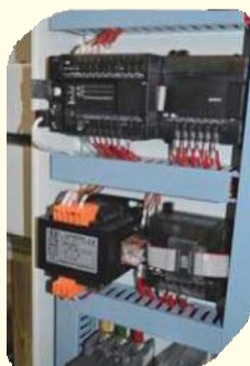
Controle PLC OMRON
